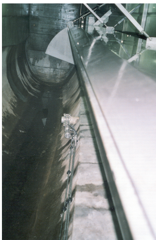
WWTP Kolben, RSW-K 11x8/4 Weir wicket closed
