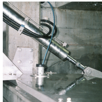
WWTP Kolben, Level probe
