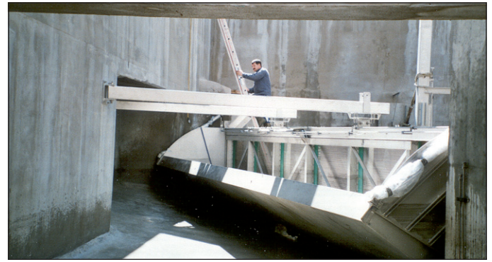
WWTP Telli at Aarau, ROMAG CSO screen RSW-K 14x8/4 (Built in phase)
