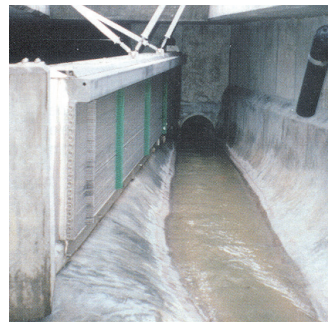
RSW 5x7/4 screen in an enclosed basin outlet
