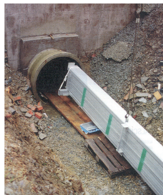
Screen admission through the outfall pipe
