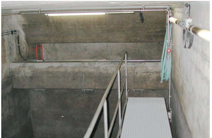
Zürich-Wollishofen sewage treatment plant, left basin half, ROMAG CSO screen RSU in the background. The hydraulic pipe for the cylinder is clearly visible. The hydraulic cylinder can just be seen above the edge of the masonry wall.
