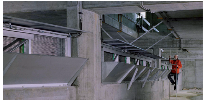
Inlet channel of the AIRE sewage treatment plant in Geneva, 3 RSW10 X 8/4, Qmax. total = 18,000 l/s View from relief sewer
